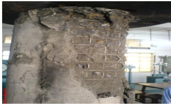
Figure: 8 Failure of weld mesh confinement
